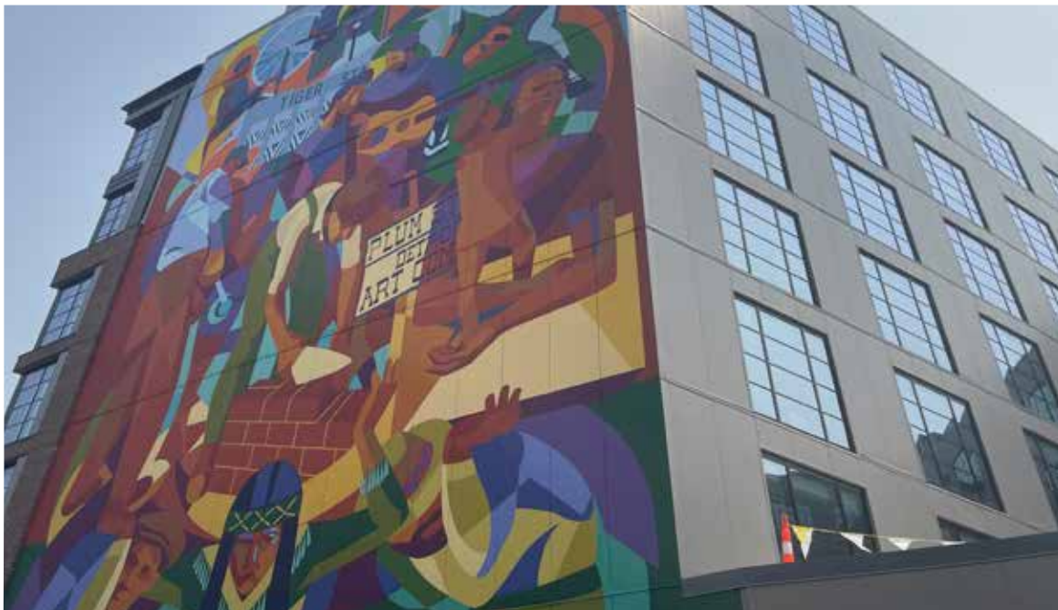
A closeup look of the hotel's metal window panels and adjacent brick work, which required special efforts by CASS workers.
