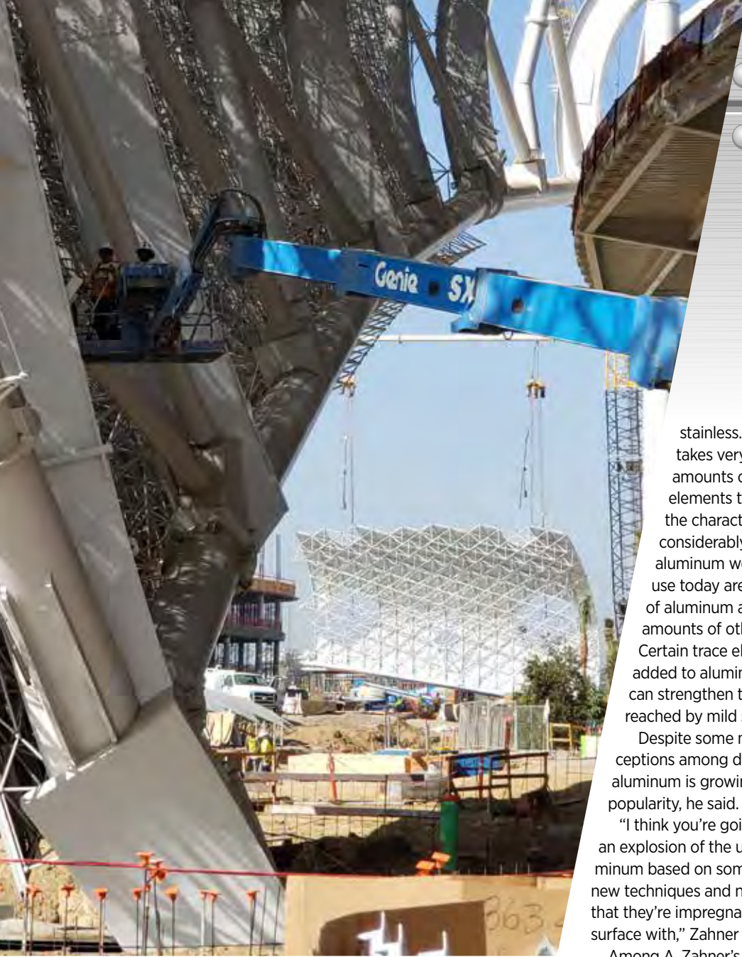
LEFT: SoFi Stadium in Inglewood Calif., home to the L.A. Rams and L.A. Chargers, has 789 perforated, custom white anodized aluminum exterior panels that were manufactured by A. Zahner.
