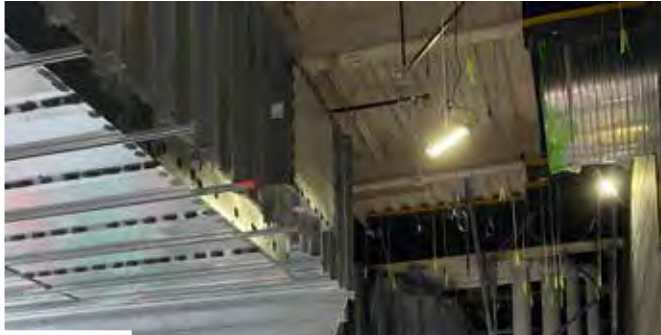
LEFT: One of the outside air ducts coming off of AHU-601. It is 142x72 with 1" liner.
